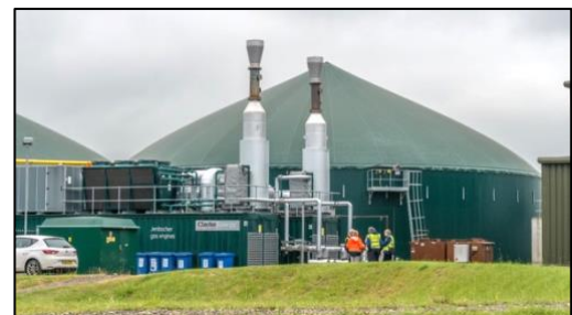
Anaerobic digester near Benson: turns our food waste into biogas
